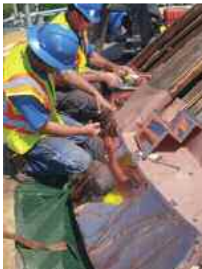
Earlier this year, crews replaced the Maine State House dome's copper with 20-ounce sheet.
